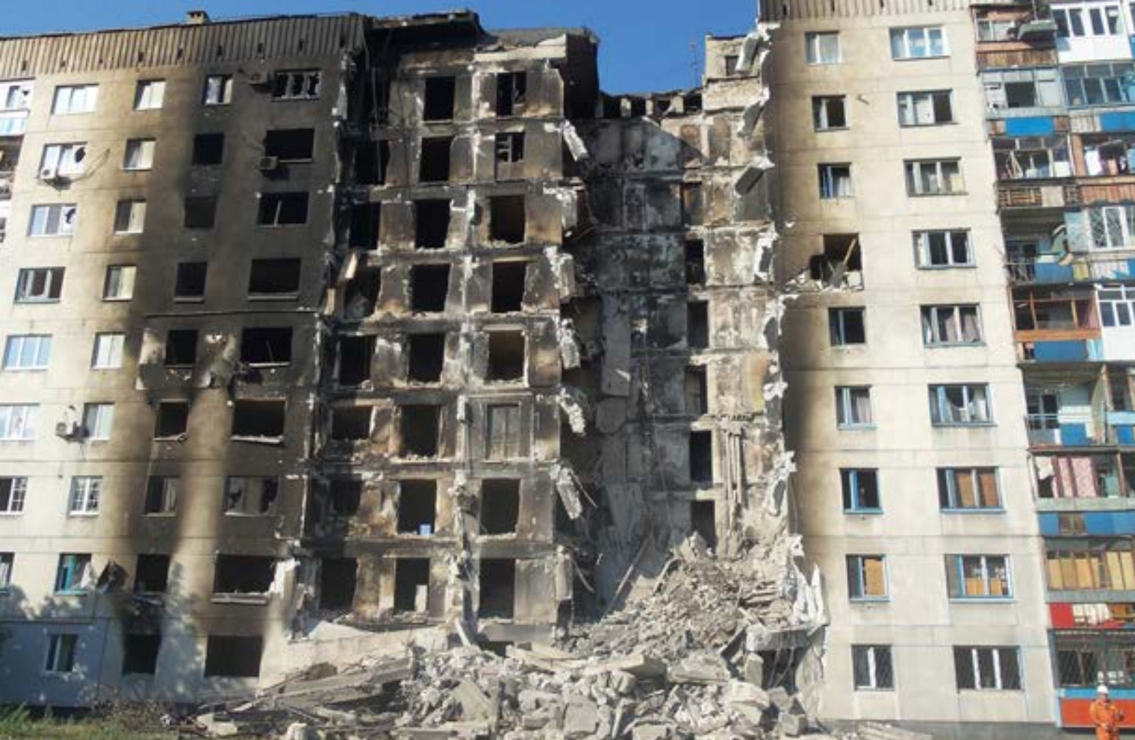
An apartment building struck by artillery fire in Lysychansk, Ukraine in August 2014. Photo credit: Wikimedia
