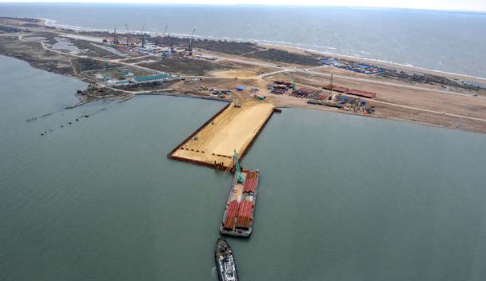
While several Ukrainian companies have initiated legal action over assets seized in Crimea, Russian authorities have proceeded with the construction of the Kerch Strait Bridge. Photo credit: The Presidential Administration of Russia
