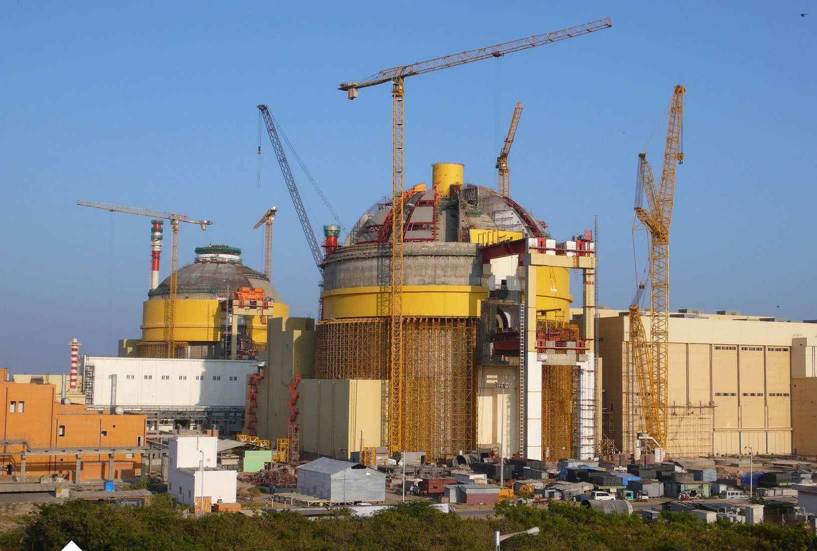
Construction of a VVER-1000 model reactor, a similar model to that planned for the Akkuyu nuclear power plant, in Koodankulam, India. Photo credit: International Atomic Energy Agency/Wikimedia.
