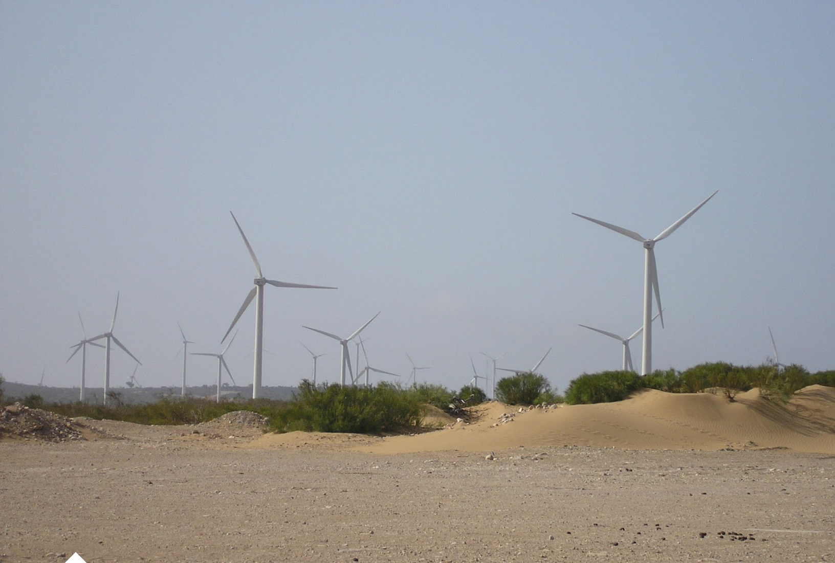
Amogdoul Wind Farm in Essaouira, Morocco. Morocco is one of several Mediterranean countries that has invested heavily in renewable energy, in order to take advantage of the basin's virtually unlimited wind and solar potential. Photo credit: Sqala/Wikimedia.
