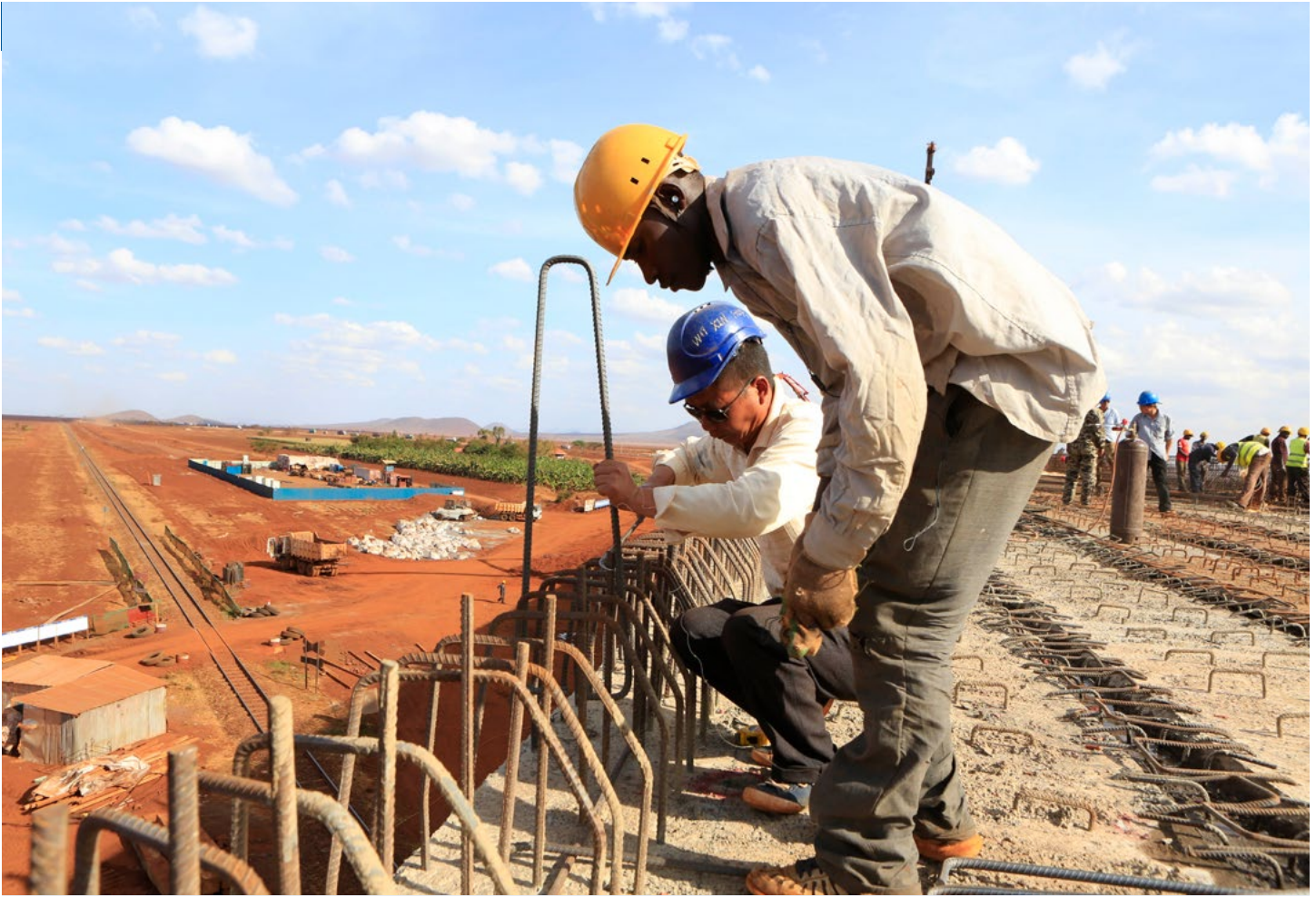
A Chinese engineer and a local construction worker work on a section of the Mombasa-Nairobi standard gauge railway (SGR) in Emali, Kenya October 10, 2015. Source: Reuters/Noor Khamis
