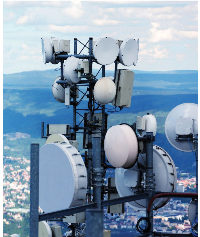
Telecommunications Antenna Source: Petr Kratochvil via Needpix
