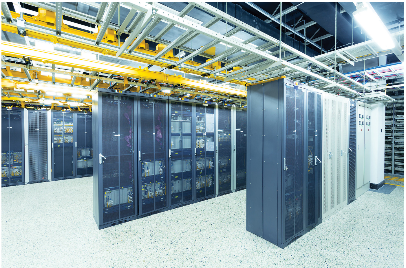
Data center room interior. Source: iStock/lovegul
