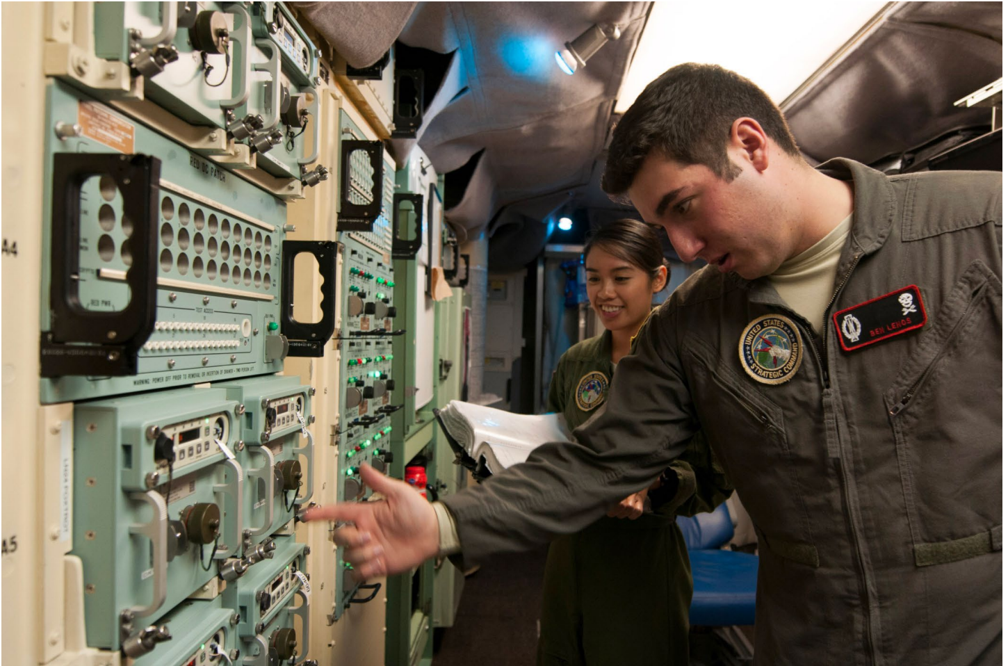
First Lt. Allia Martinez, 320th Missile Squadron missile combat crew commander and 2nd Lt. Benjamin Lenos, 320th MS deputy combat crew commander perform checks on the strategic automated command and control system in a launch control center at F.E. Warren Air Force Base, Wyo., Nov. 6, 2016. The 90th Missile Wing sustains 150 Minuteman III ICBMs and the associated launch facilities that cover 9,600 square miles across three states. (U.S. Air Force photo by Staff Sgt. Christopher Ruano). https://tinyurl.com/uzjheawb .
