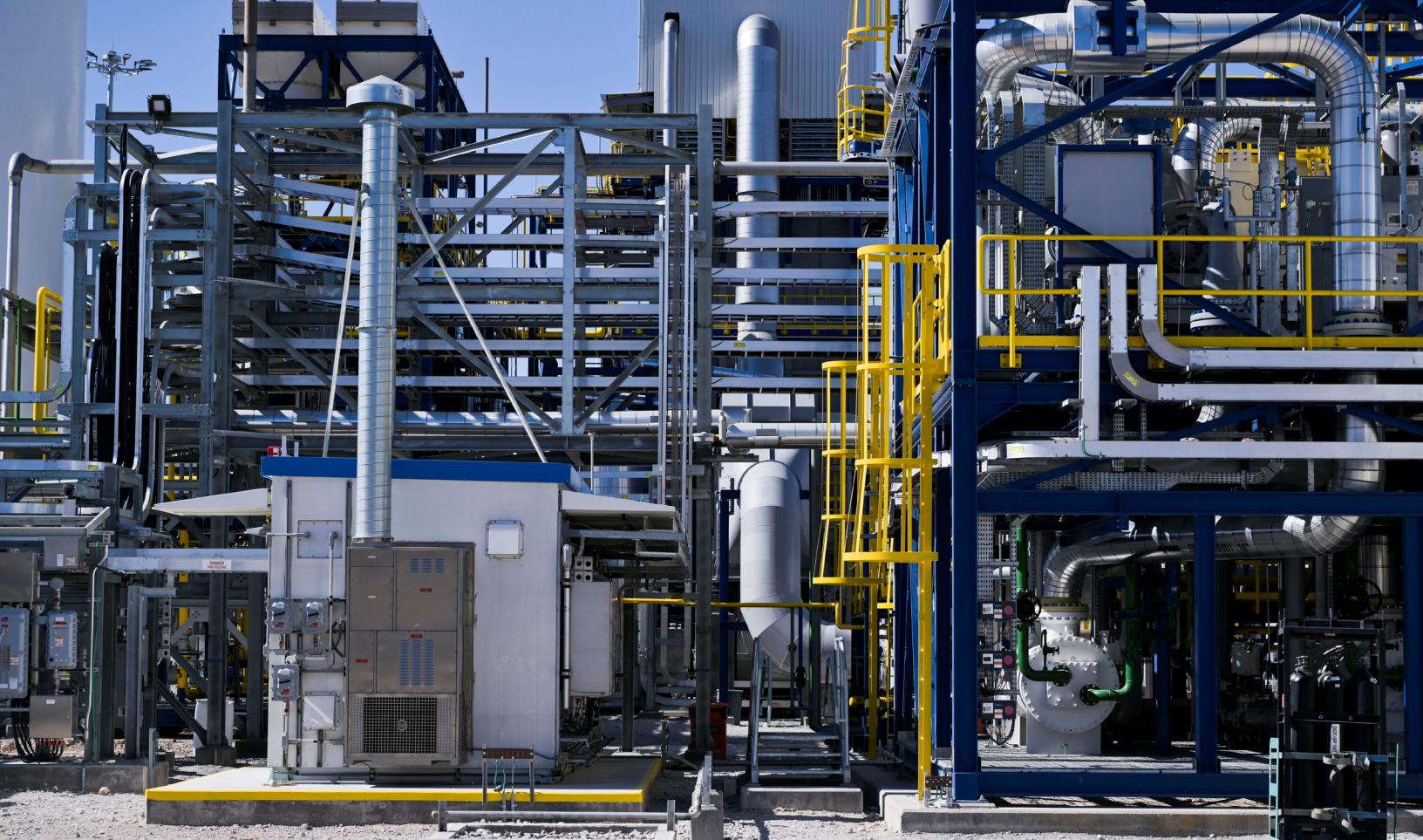
Air Liquide opens its North Las Vegas Hydrogen Production facility in Las Vegas, Nevada, May 24, 2022. REUTERS/Bridget Bennett
