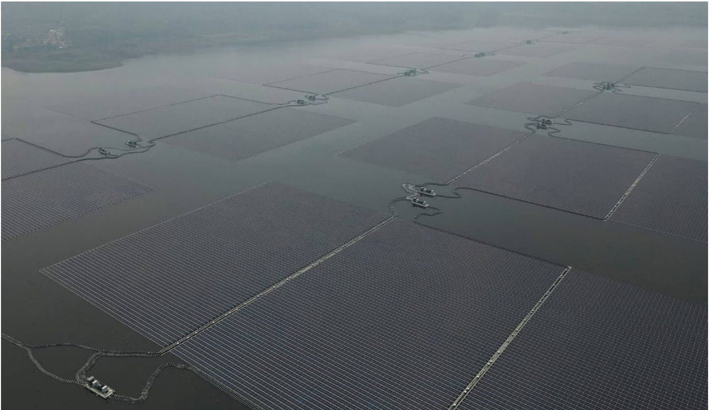
A view shows solar panels of the 192 megawatt peak (MWp) floating solar power plant built on Cirata dam, that was developed by PLN Nusantara Power, a unit of Indonesia's state utility company Perusahaan Listrik Negara (PLN) and United Arab Emirates renewable energy company Masdar, a unit of Mubadala Investment Company, in Purwakarta, West Java province, Indonesia, November 9, 2023. Source: REUTERS/Willy Kurniawan
