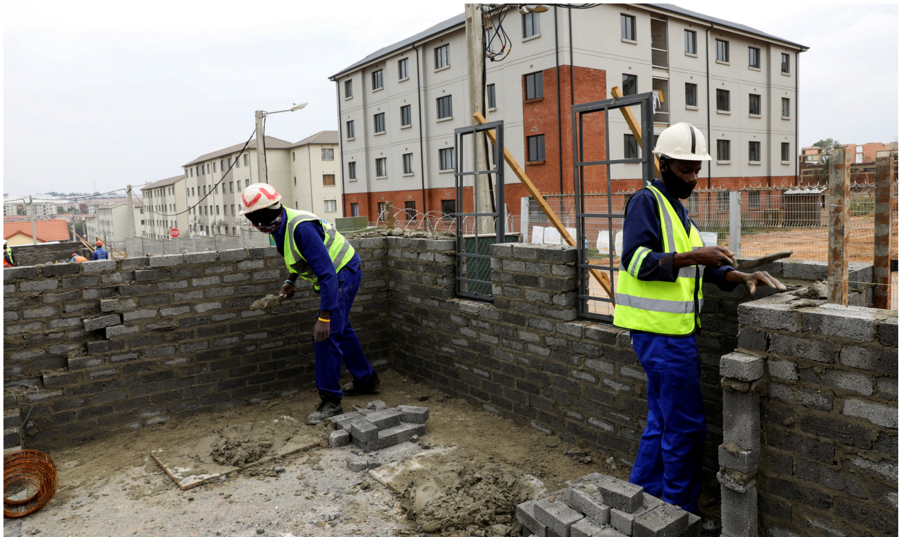
Workers are seen building housing units at a construction site as coronavirus disease (COVID-19) lockdown regulations ease in Fleurhof, near Johannesburg, South Africa, October 6, 2020. REUTERS/Siphiwe Sibeko
