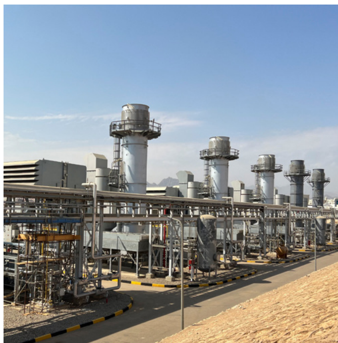
Electricity generation turbines partially fuelled by green hydrogen in Sharm El-Sheikh, Egypt, October 20, 2022. REUTERS/Sayed Sheasha.
