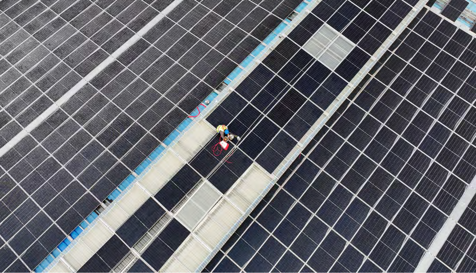
Construction workers install photovoltaic modules on the roof of the factory building of Jiangsu Beijiali Machinery Technology Co., Ltd. in Hai'an Industrial Park, Jiangsu Province, China, on April 1, 2026.
