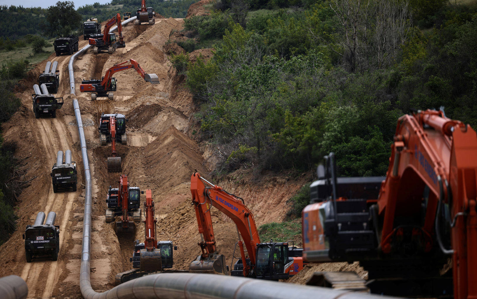
Excavators work on the site of the construction of the Vertical Gas Corridor, near Mikrevo, Bulgaria. REUTERS/Stoyan Nenov
