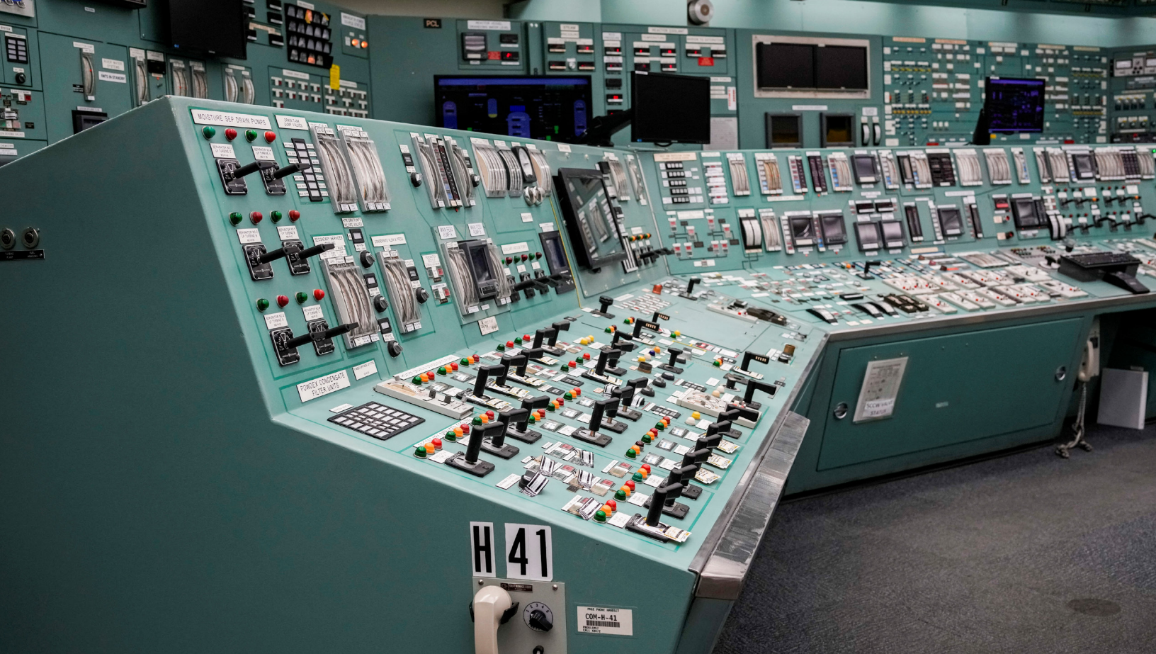
The control room of the Crane Clean Energy Center, formerly called the Three Mile Island Nuclear Station. REUTERS/Eduardo Munoz
